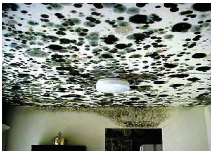
Figure 5.1. Mold Growth in the Home
